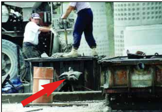
US-1600 with wedge on culvert form. (Notice a rubber sheet covers vibrator and protects it from concrete spill.)
