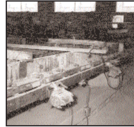
US-900 with Wedge Bracket on precast mold
